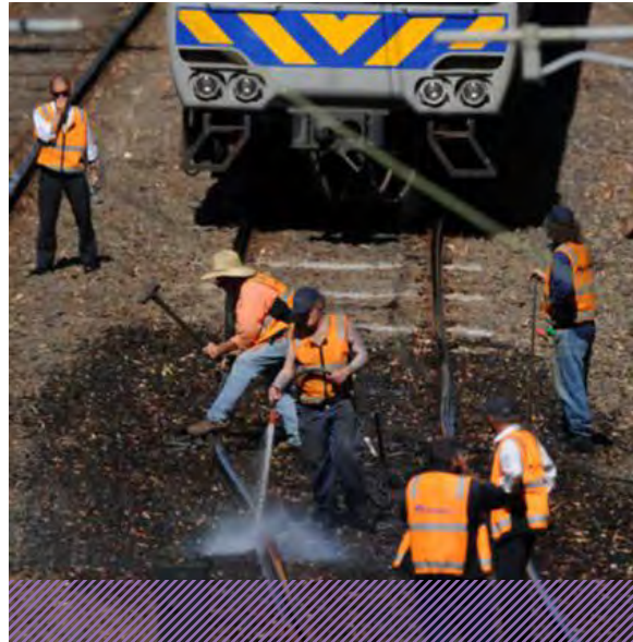
Figure 41: Maintenance officers in Melbourne work on train tracks that buckled under the extreme heat of 28 January 2009.
