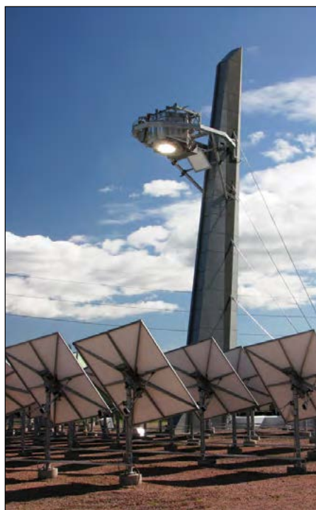
Figure 4: CSIRO's SolarGas™ reactor in Newcastle, New South Wales.
